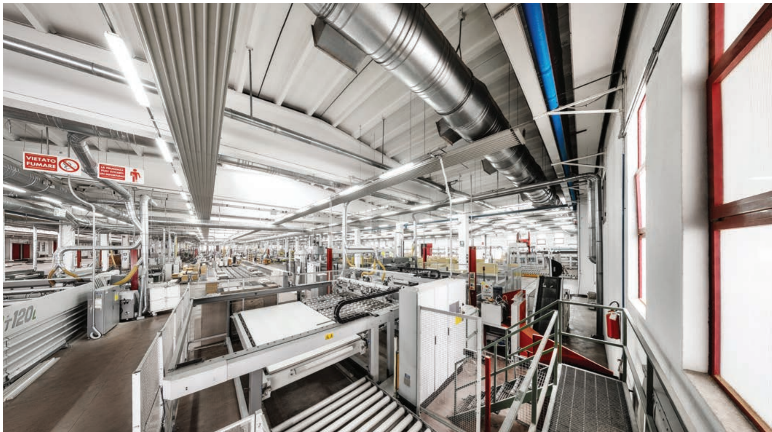
Panel production line/
